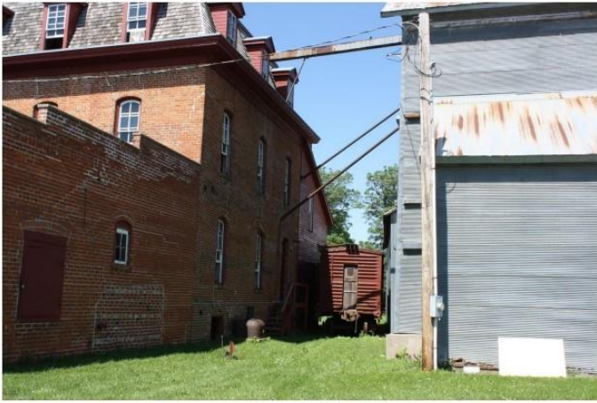
12. View showing relationship and physical connection between brick mill building and elevators looking northwest.
